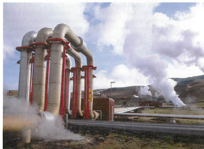
▼ FIGURE 9-47 GEOTHERMAL Geothermal plant near Krafla, Iceland.
